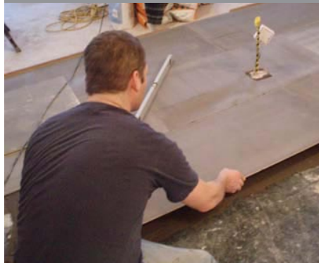
Underfloor Heating Insulation
