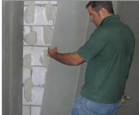
Dot and Dab to Damp Basements
